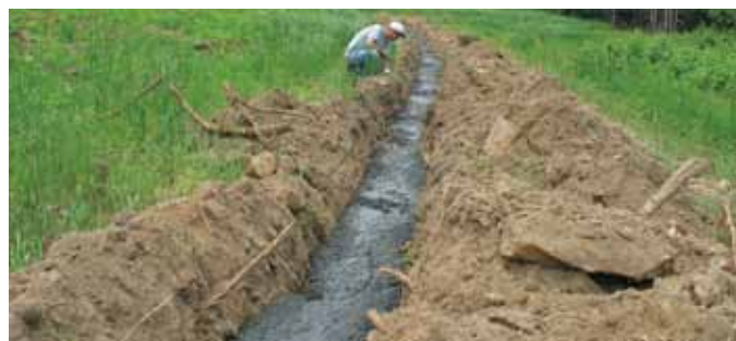
A trench was dug around the existing copper grounding ring and backfilled with HCC (photo courtesy of We Energies)
