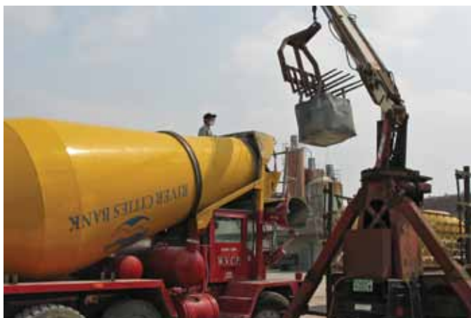
HCFA is added to a concrete mixture. This batch was used for a grounding contact for a telecommunications tower in Rudolph, WI. It was the first practical application of electrically conductive high-carbon fly ash concrete (photo courtesy of We Energies)
